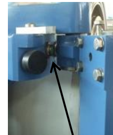
Limit switch Filtrate Housing open
