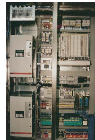
Manufactured inverter cabinet
